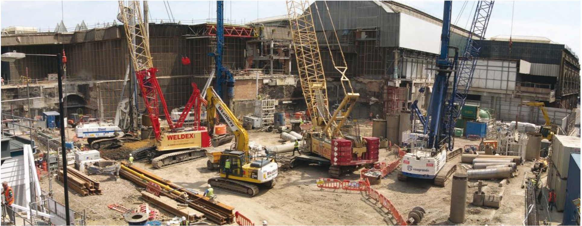
Piling for the building began in March 2009 following the demolition of the 26-storey Southwark Towers. A view of the Sharda building construction site in June 2009
